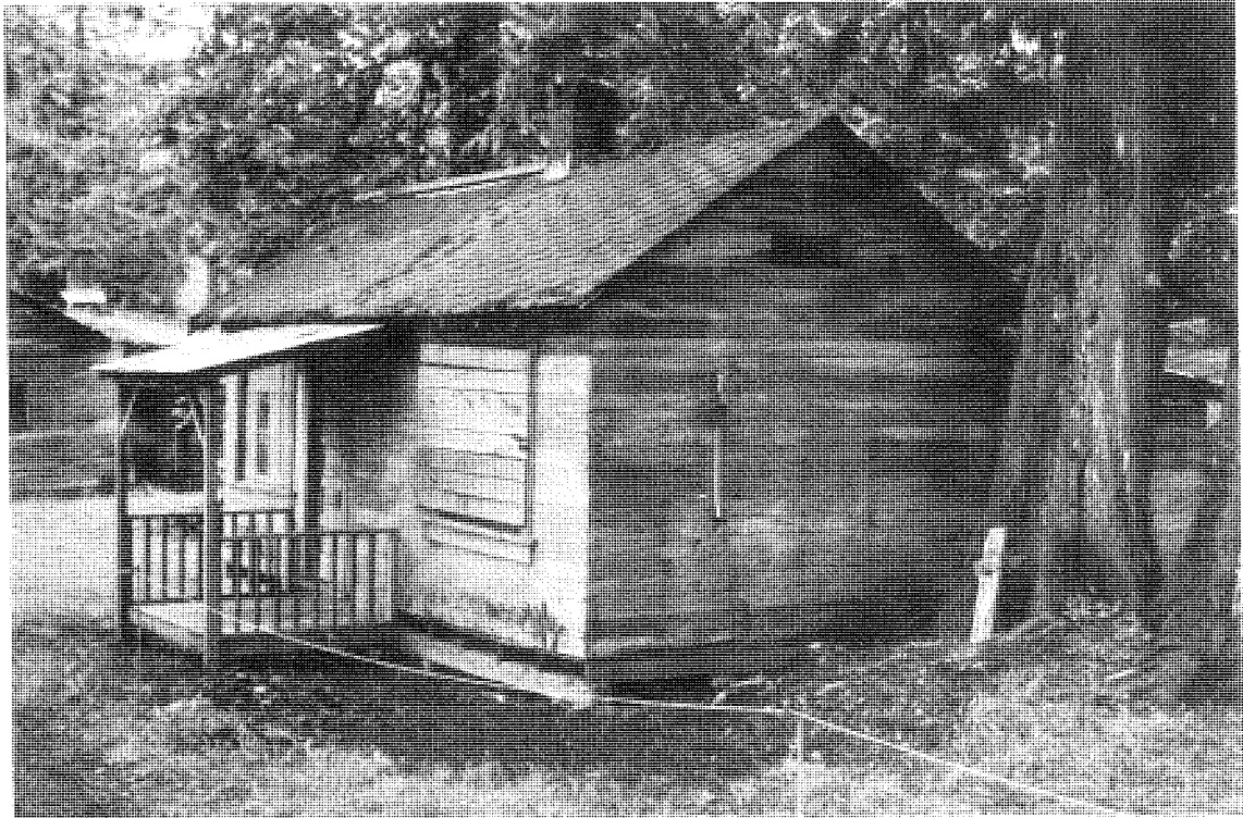
Bookkeeper's House and Office (No. 22) as found, January 1990, and after stabilization, July 1992. Note new sills and floor joists, removal of vegetation around the house, and removal of organic growth from the roof.
